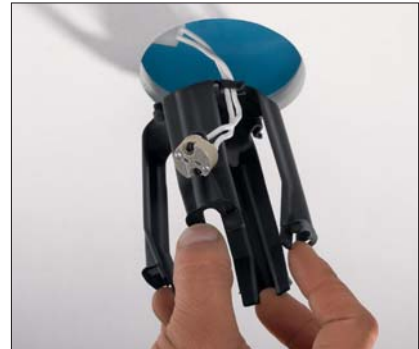
Fix the supply cable in place, push the mounting clips together, and insert in the ceiling cavity.
